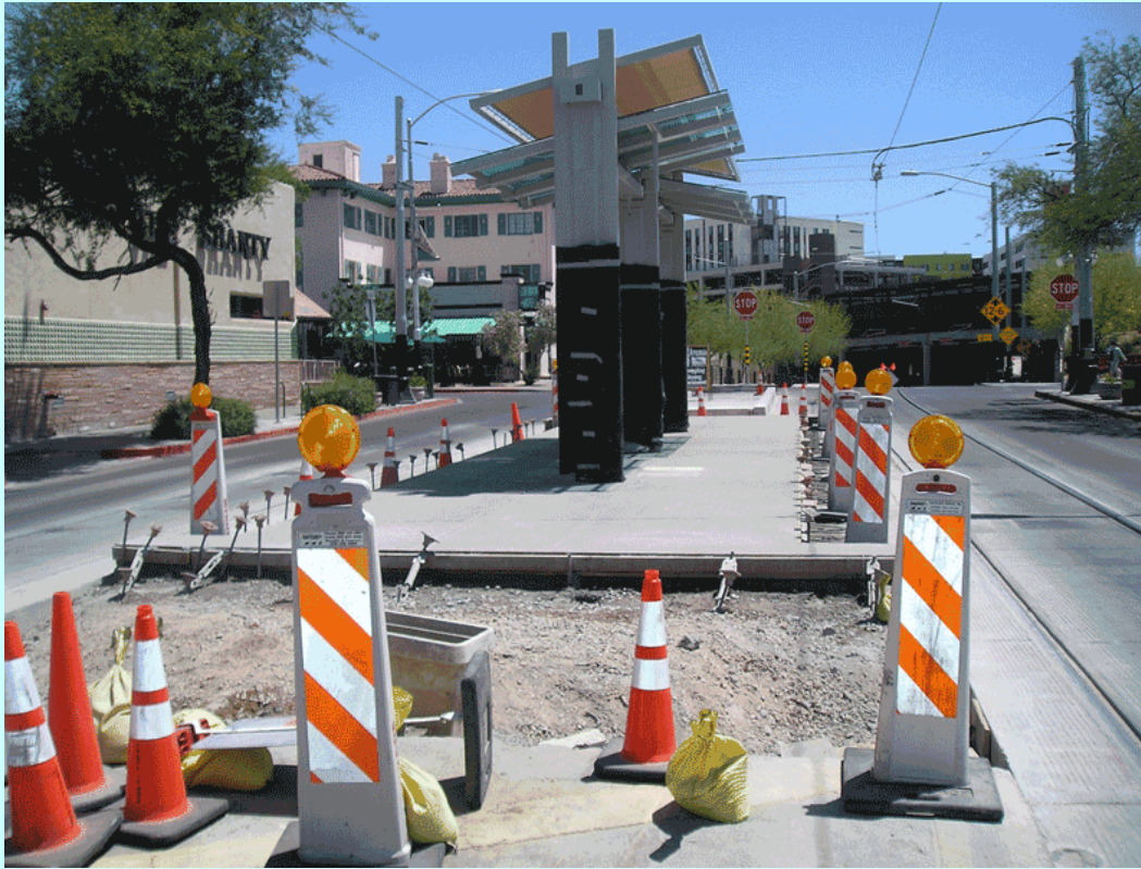
Figure 6 - Rebuilt Streetcar Platform. First installation was to high to allow wheelchair ramp deployment from streetcars.
